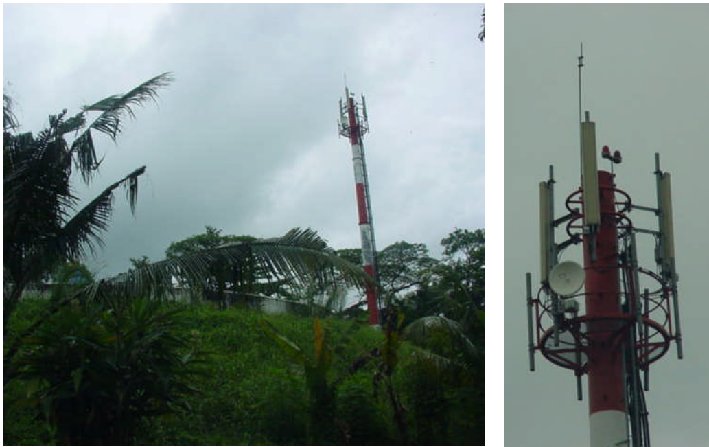
Figure 4. Photograph of the Mobile Telephone Base Station Tower at Kg.Tarom
